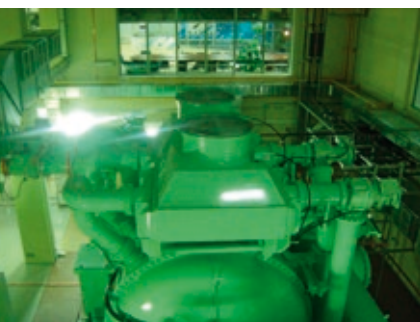
Gas insulated transformer in the Skolkovo substation
