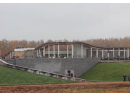
The Skolkovo substation
